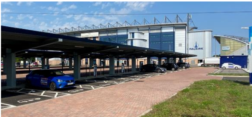
Falkirk Stadium - Scotland's largest EV hub (26 bay)
